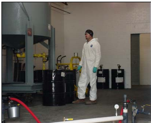
INJECTION AREA WITHIN CHEMICAL TRANSFER ROOM OF FACILITY
